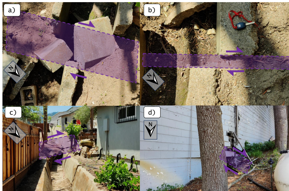
Figure 1.7: Damaged drainage gully and wall at the Cienega Winery, Cienega Rd, Hollister, CA. a), b) & c) Drainage gully offset by right lateral creep. d) Damage to the NW wall of the winery building due to right lateral creep.
