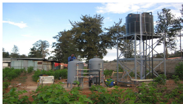
Fig. 27 An example of the Manna Energy Limited water treatment system. The system is installed in-line with existing water pipes. On the right is an elevated backwash tank. In the center is a gravel filter and a pressurized sand filter. On the left is the solar photovoltaic-powered UV system.
