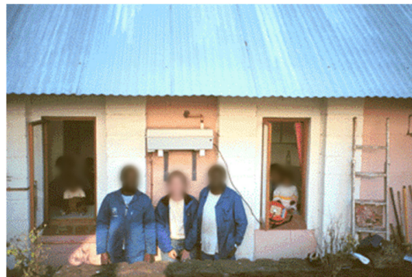
Fig. 29 UV Waterworks 2.0 unit installed on the exterior wall of the kitchen at the Lily of the Valley HIV-Hospice near Durban, South Africa.
