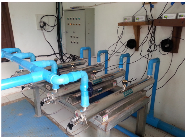
Fig. 15 UV disinfection system.
