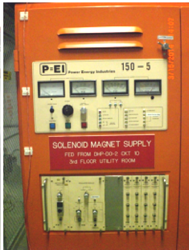
(b) Control Panel
