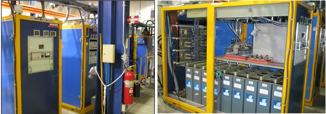
Figure 7.18: Existing lens and PMAG power supplies at AP0.
