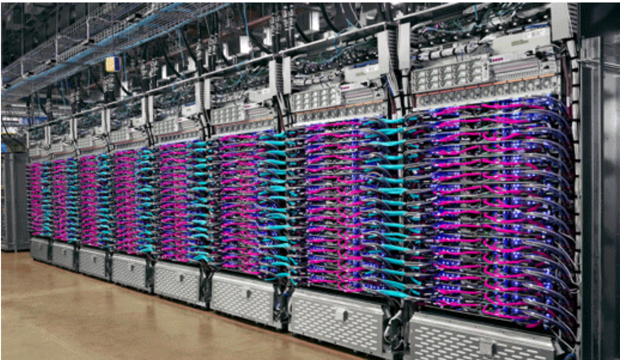
Figure 4.4: An aisle of rack-based servers containing TPUs. Source: Google.
