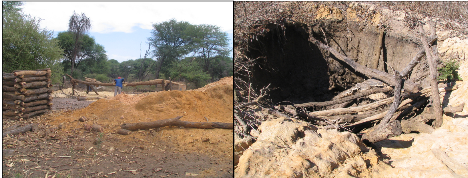
Plate 6.1. A well at the Kwarongo cattlepost: (i) under construction, photo taken in October 2005 (left); and (ii) six months after it collapsed, photo taken in June 2006 (right). Source: fieldwork.
