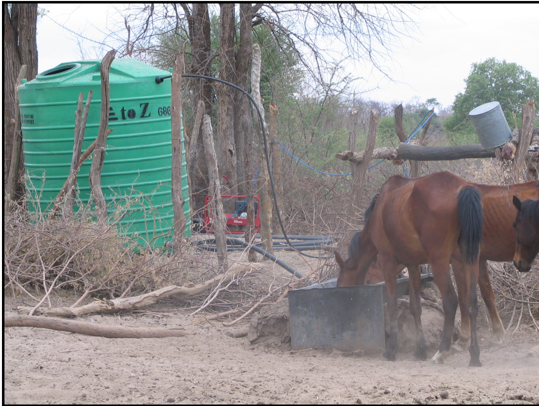
Plate 5.1. The mechanisation of cattlepost wells in the Chukumuchu rangelands typically consisting of a small electric water pump powered by a petrol or diesel generator which supplies water to a 2000 litre plastic storage tank
