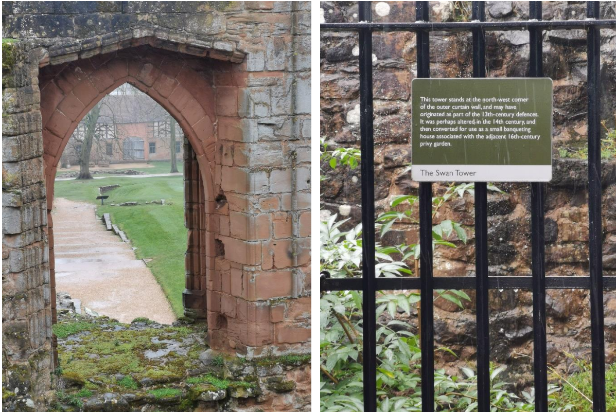
Figure 2.8 (left) Grass and mosses colonising inaccessible floor surface in the Great Hall, and (right) Self-set Ash tree behind a permanent screen in the Swan Tower. Images © Author
