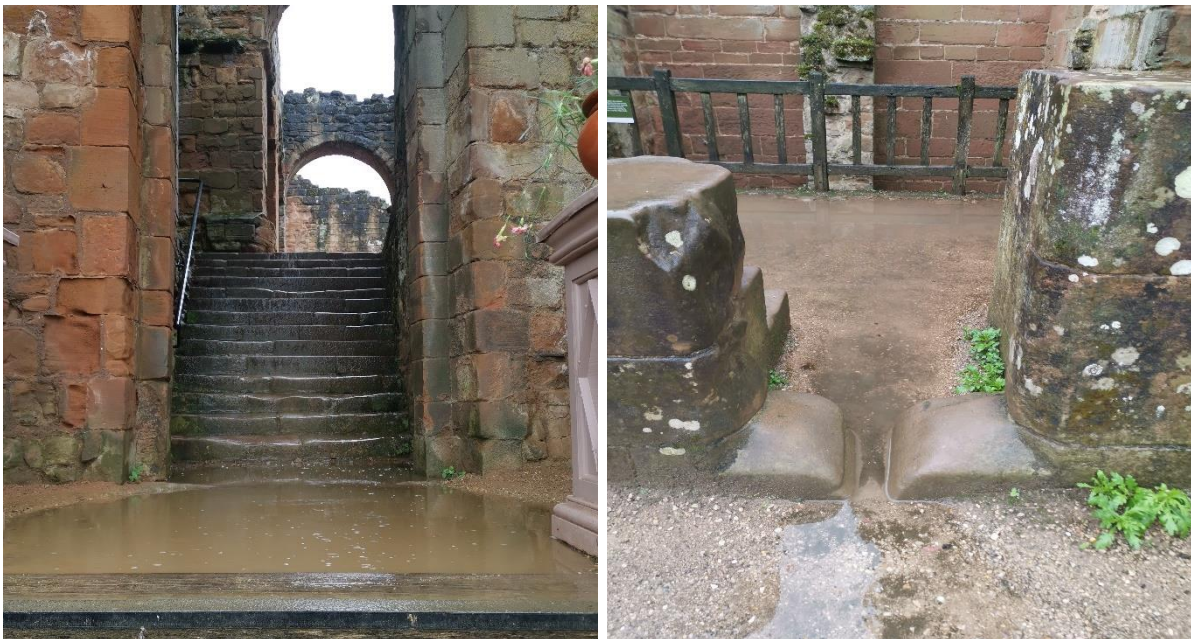
Figure 2.7 (left) Pooling rainwater in the north entrance to the Keep, and (right) the combined effects of water and footfall erosion on a doorway stone, State Apartments. Images © Author
