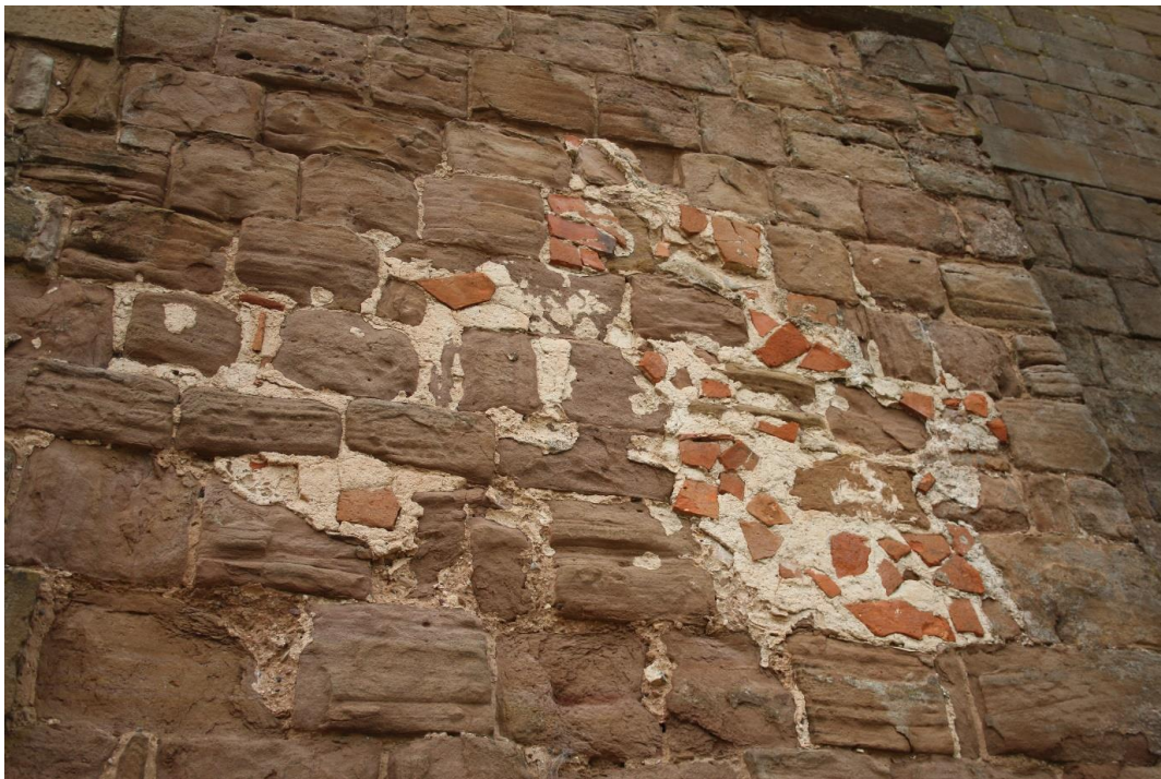
Figure 2.11 Modern stabilisation and structural repairs, using brick and concrete mortar to infill lost stonework. Image © Author
