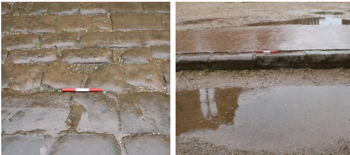
Figure 2.14 Left: Type 3 floor surface historically covered but now exposed to environmental erosion. Right: Type 4, modern stone, concrete, and aggregate mix. This setting is adjacent to the earliest extant area of the castle complex (12 th Century). Scale 0.3m. Images © Author
