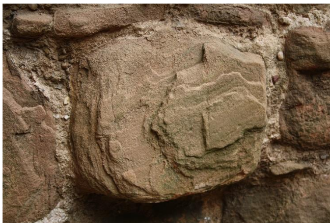
Figure 2.9 Delamination of structural stone, located in the Great Hall Image © Author
