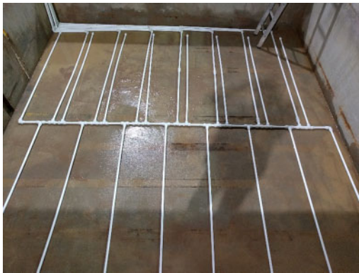
Figure 7. Perforated pipes installed in the pit section of the Fast Flow Facility.
