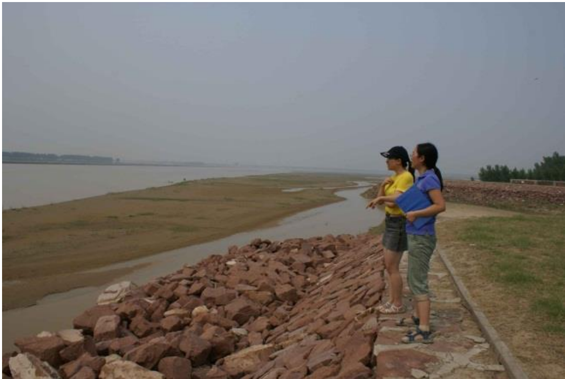
b. Flood defense infrastructure (levees) built in 2005 along LYR, with a length of 300km
