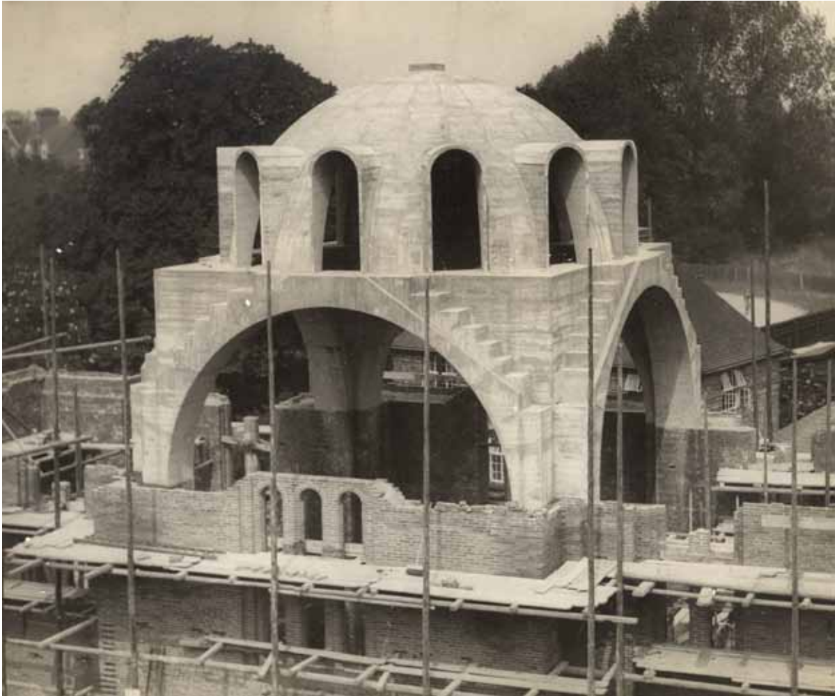
Fig. 1.36 Photograph of the Lady Margaret Hall Chapel under construction, showing the concrete dome, c. 1932. RIBA.
