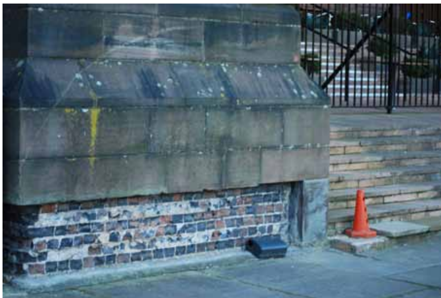
Fig. 3.55 Minor damage to north porch of Liverpool Cathedral reveals the relationship between the stone veneer and the structural brick masonry beneath. Author, 2012.
