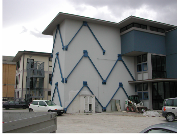
Figure 2.33: Elastomeric dampers used for seismic retrofit in the Gentile-Fermi School in Fabriano [8]
