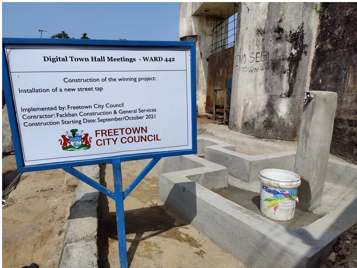
FIGURE A2. Street Tap Implemented in Ward 442
