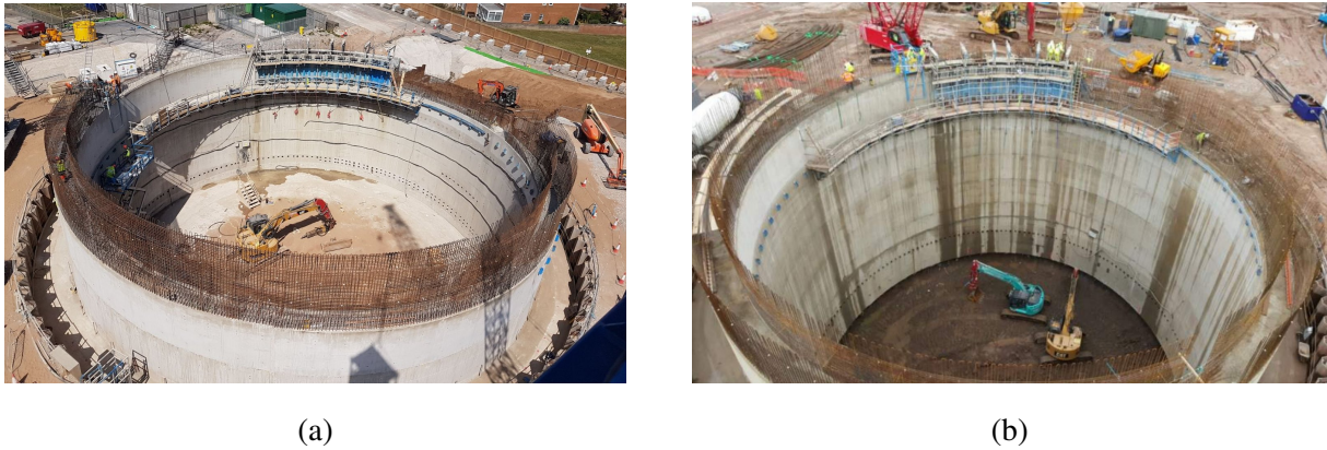
Figure 1.4 Construction of a 32 m internal diameter open caisson shaft by Ward & Burke Construction Ltd for an underground pumping station in Blackpool, UK: a) wall casting pre-excitation, b) structure sunk into the ground post-excitation
