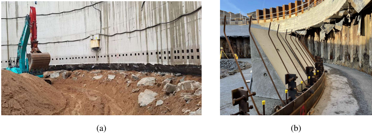
Figure 7.8 Caisson shaft cutting face formation: a) Breaking out a bearing pad prior to sinking, b) removable pre-cast blocks
