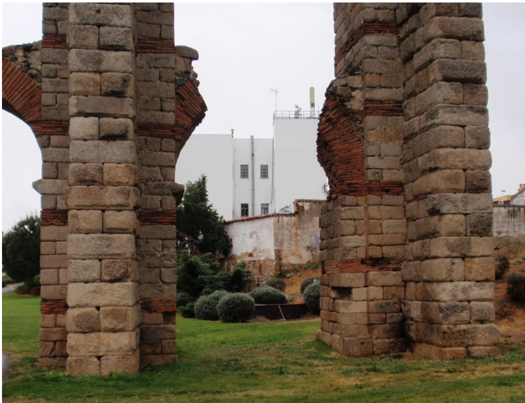
Fig. 3.38 – Mérida: Los Milagros aqueduct: late repair in which an extra reinforcement has been added to the intrados of the pier on the right, on which a new brick arch was built, as evident from the dissimilar impost heights at both ends of the arch.
