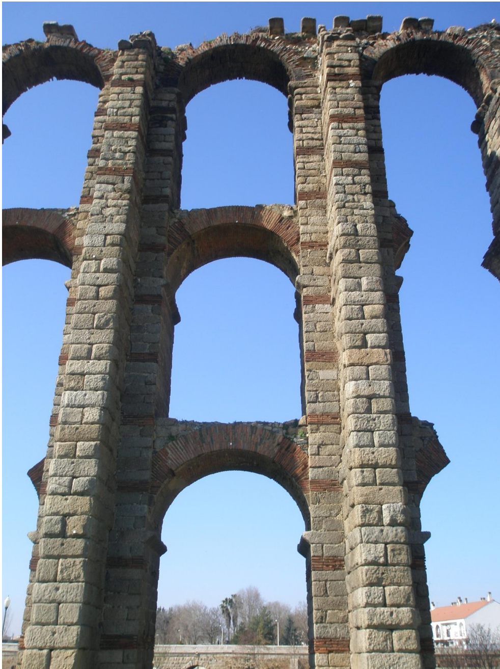
Fig. 3.32 – Mérida: Los Milagros aqueduct: piers sustained by three tiers of brick arches and extra buttresses (photo by Sofía Benavente).
