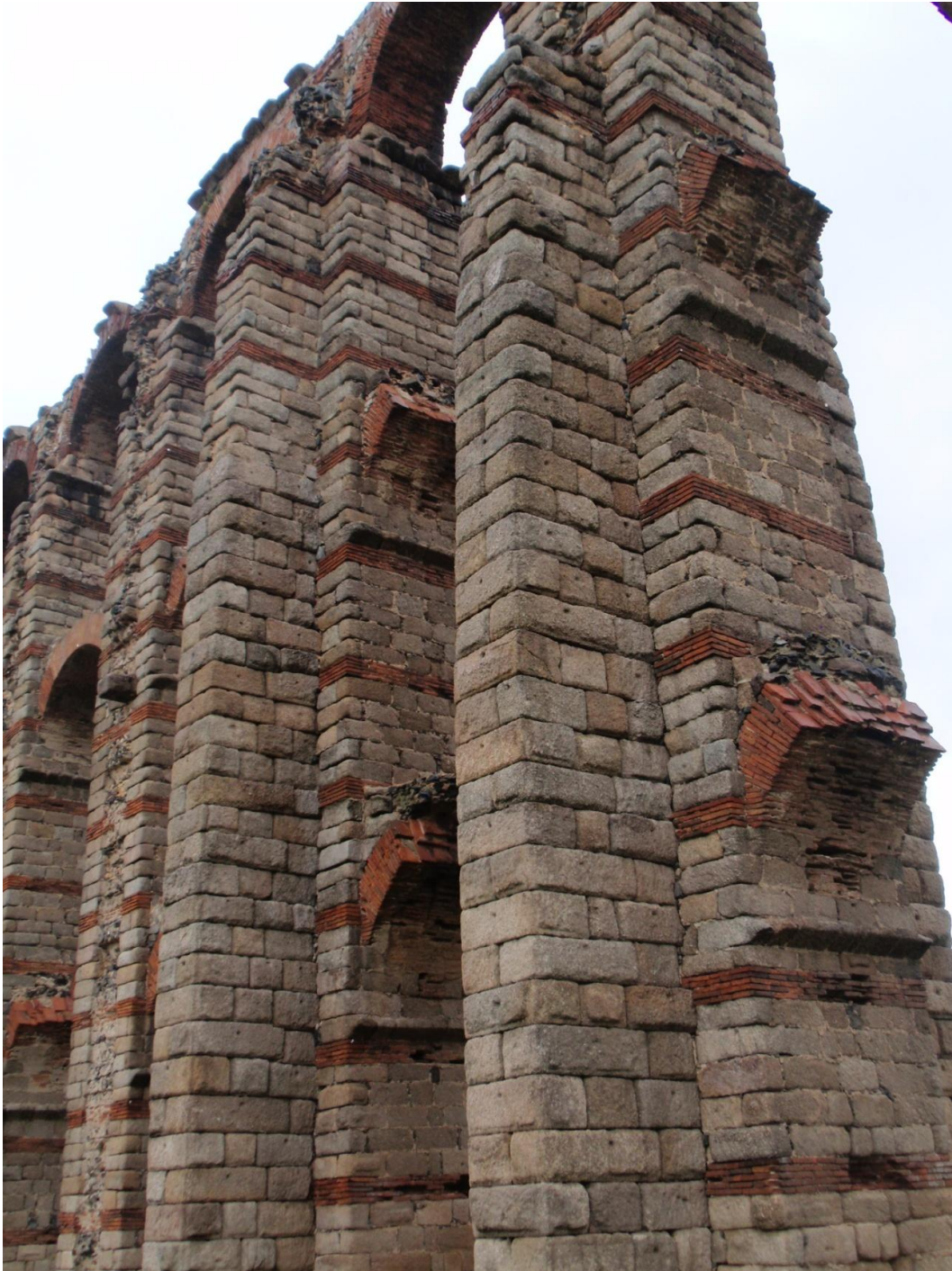
Fig. 2.1 – Mérida, Proserpina aqueduct: Buttresses added to the pillars built in a different technique indicate later repairs.
