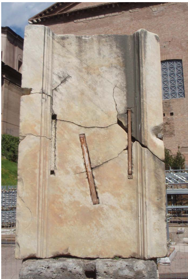
Fig.11 LSA 1363. The base for a statue to the Fides and Virtus of the emperor's armies, erected in the middle of Rome's Forum in 406. Note the cracks in the marble, the repair-clamps, and the difference between the mouldings on the right and left of the base (the fillet of stone on the right has a profile with a convex curve, since it was originally the top edge of a base for an equestrian statue).
