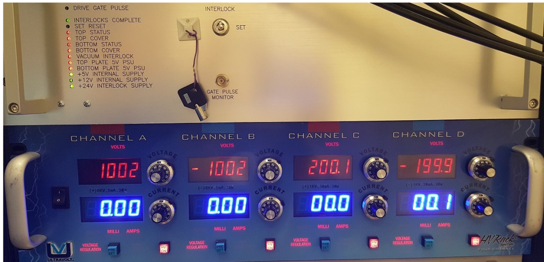
Figure 7.15: Chopper drive electronics crate (top) and UltraVolt four-channel high voltage power supply crate (bottom).
