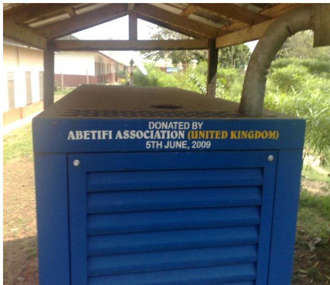
Plate 6.3.1 Power generation equipment
