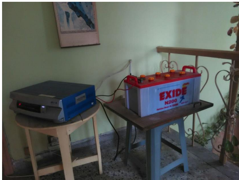
Figure 5.2 UPS and battery – photograph by Ayah
