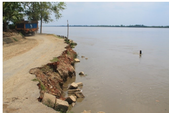
b. Riverbank erosion damaging embankment (Polder 30)
