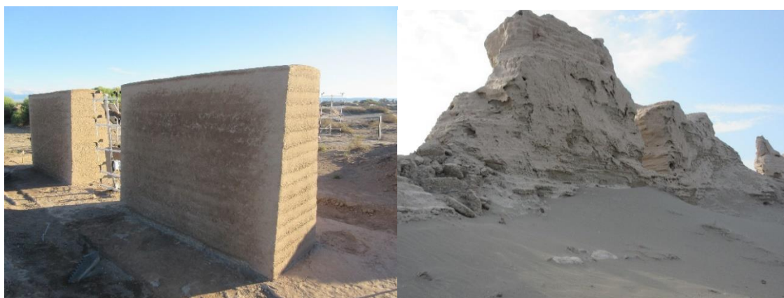
Figure C.13: The impact of rain on a) test wall 24 hours after a storm event, and b) on the historic walls
