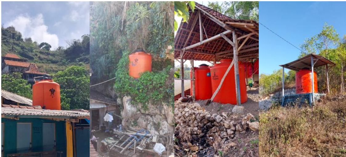
Figure 4.1.4.14 Water Storage Tanks
