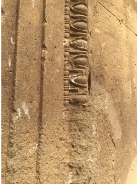
Figure 3.20: Detail of the doorframe of the main entrance of the Chetinyova (4) tomb
